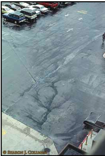
Parking lot oil entering storm drain.
